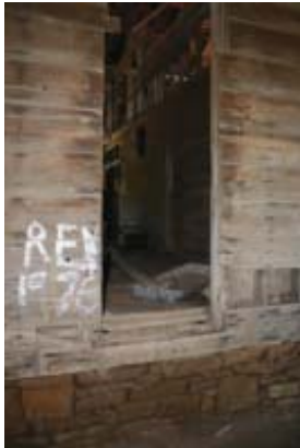
Sac and Fox Mission Building northeast wall, Ford, 08/02/2011.
