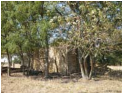
Havana Stage Station. Looking SW at the east (left) and north (right) elevations of the station. 08/09/2012. KSHS/Hoard, Bob.
