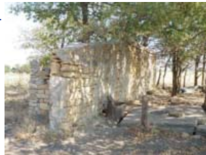
Havana Stage Station. Looking NNW at east elevation of station. 08/09/2012. KSHS/Hoard, Bob.
